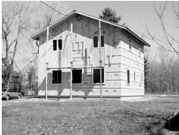
Locally harvested and milled siding was applied board and batten-style over 2 inches of EPS.
