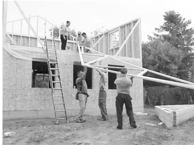
Energy trusses donated by a local company are installed by Habitat volunteers.
