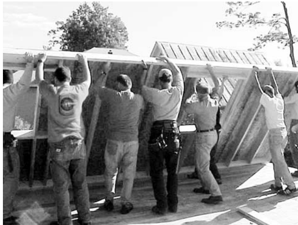
Habitat volunteers lift a wall section into place. Studs were spaced on 24-inch centers to reduce heat loss and lumber use.
