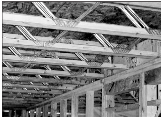
The IRC 2003 (R-502.12) requires that "draftstops" be installed to separate floor/ceiling assemblies into "approximately equal areas" not exceeding 1,000 square feet. Dropped ceilings and open web truss floor systems are specifically mentioned as the primary target areas for draft stopping.
