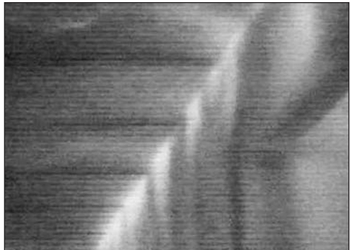
An infrared scan taken during the summer reveals air leakage at the top plate of an interior second-story partition. Much of this leakage could have been prevented by the application of a continuous fat bead of caulk along the inside edge of the double top plate as part of the drywall hanging process.
