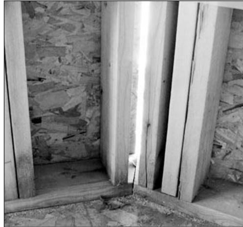
Exterior OSB sheathing is allowed to float across framing of a bay wall. If this nearly one-inch, floor-to-ceiling gap is left unsealed, the builder should expect a comfort-related callback.
