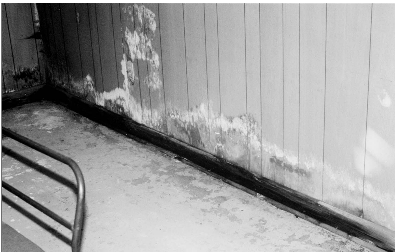
Don't even think about sleeping in a basement with such extensive moisture damage.
