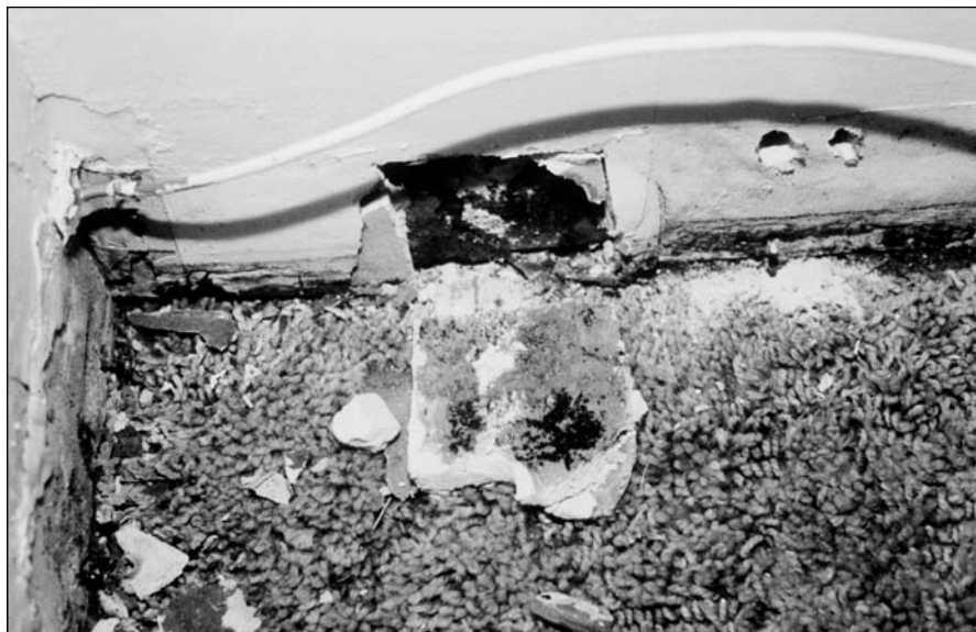
Although this carpet was dry, mold was found inside the basement wall.
