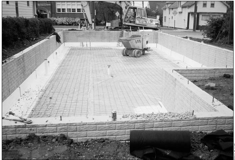
Two-inch foam panels under the slab and up the walls of the crawlspace not only reduce heat loss, but also greatly reduce the chance of condensate forming on the slab.
