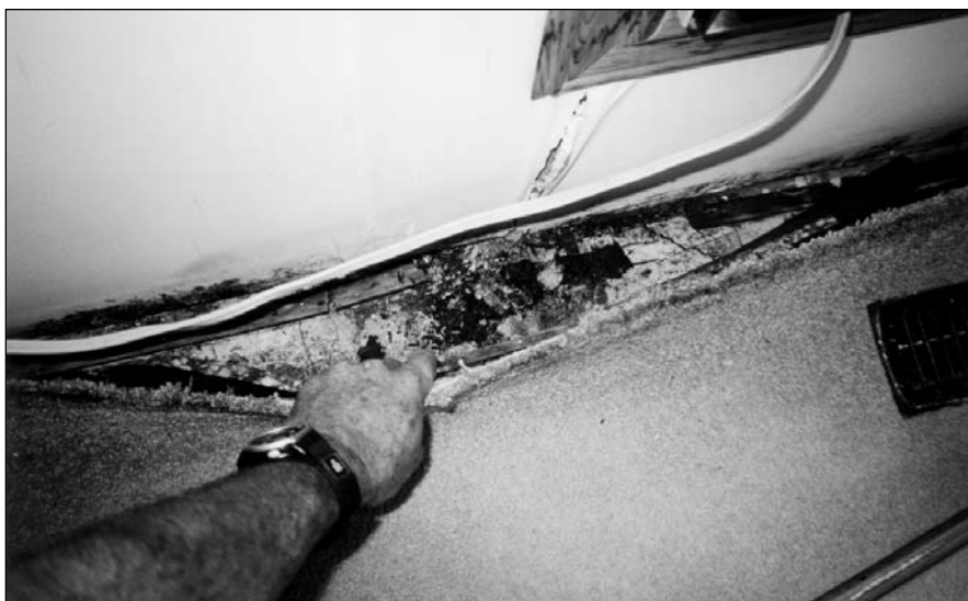
Pulling back carpet reveals the heart of the mold problem.
