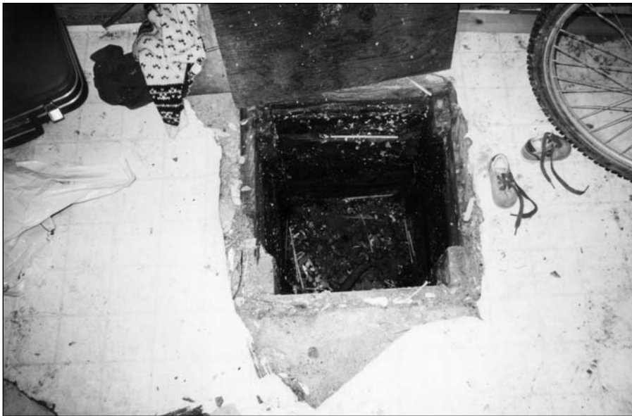
Located in a heavily trafficked area, this wooden sump pit has provided an optimal environment for mold growth.
